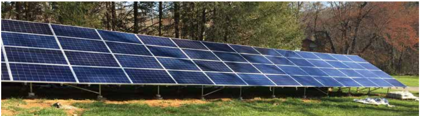
New solar panels at the Yearly Meeting office
